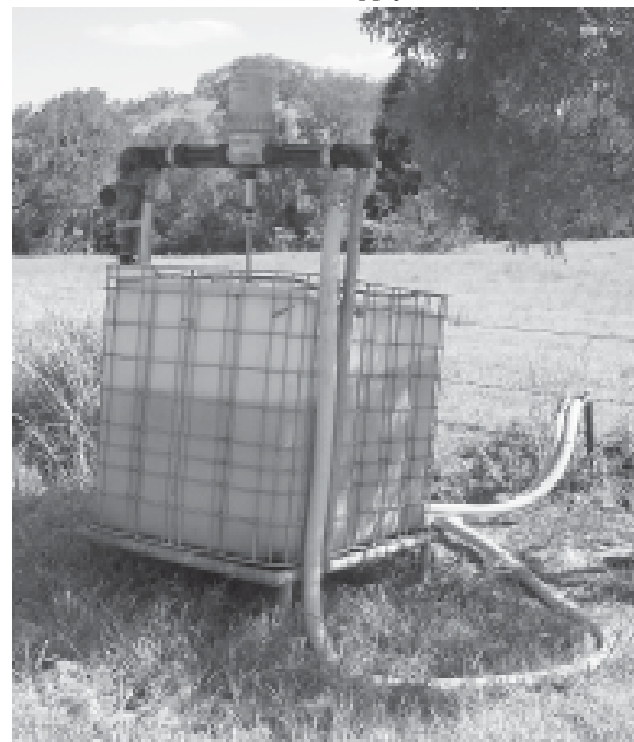
Dispenser meters nitrogen supplement into the piped water supply
